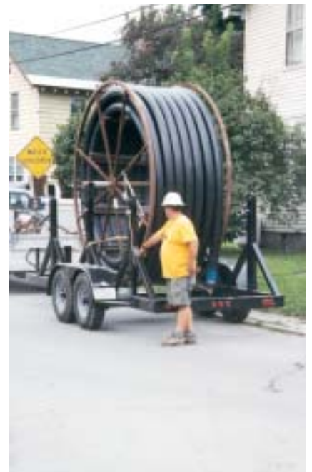
A 500-foot coil of 5-inch HDPE conduit stands ready to be fused with a second coil.
