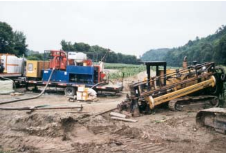
Below: Mud recycler, center, is connected in a closed circuit with Vermeer drill at right, while at far left is STS 1500 mud mixer.
